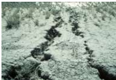
Figure 4-1 An example of eroded dike slopes.
