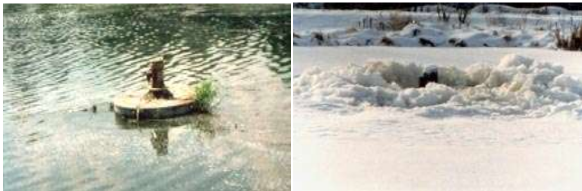
Figure 3-3. Floating aerators in summer and winter operation.
